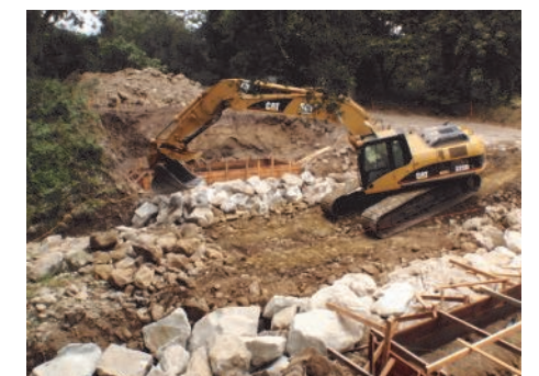
SHAW CONTRACTING INC WORKING TO PLACE LARGE ROCK AROUND THE BRIDGE ABUTMENT FORMS
