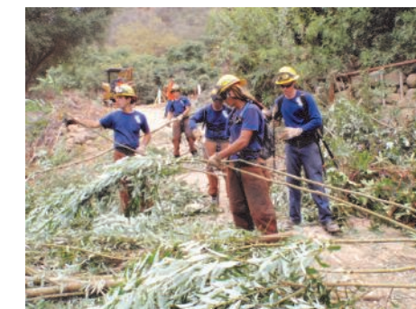
CCC CORP MEMBERS WORKING TO SALVAGE WILLOW POLES FROM THE SITE PRIOR TO CONSTRUCTION
