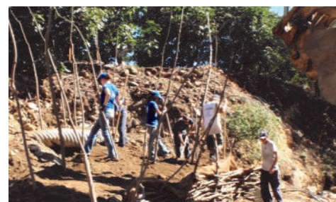
WSP MEMBERS WORKING WITH THE CALIFORNIA CONSERVATION CORPS TO BUILD A WILLOW WATTLE FENCE
