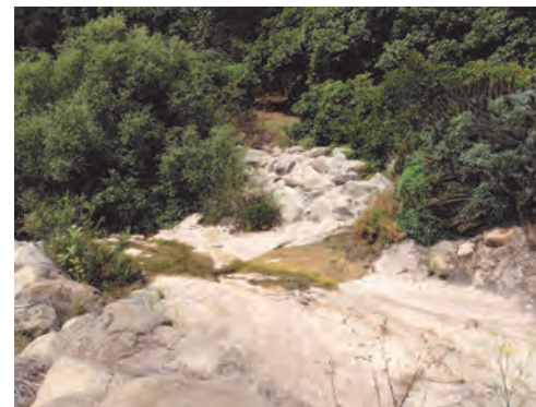
VIEW OF CONCRETE IN THE CREEK WHICH INHIBITS STEELHEAD MIGRATION.
