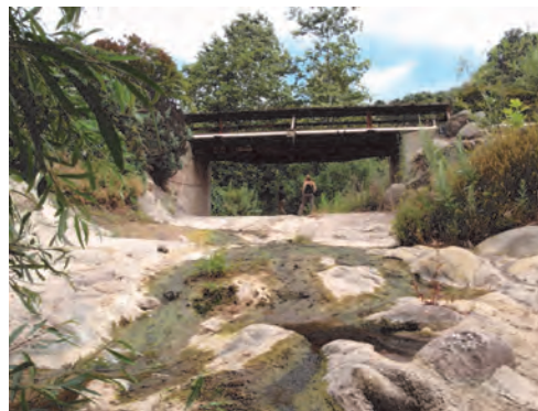
THE CURRENT PINKHAM CROSSING IS A COMPLETE BARRIER TO STEELHEAD PASSAGE.
