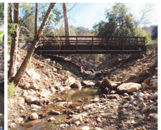
AFTER UPSTREAM VIEW OF REMOVED BARRIER AND NEWLY INSTALLED BRIDGE AND POOLS.
