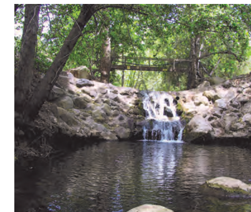
BEFORE UPSTREAM VIEW OF THE BARRIER TO STEELHEAD MIGRATION WHICH WAS REMOVED AS PART OF THIS PROJECT.
