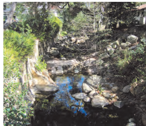
LOOKING UPSTREAM FROM THE PEDESTRIAN BRIDGE AT THE WALL AND CONCRETE APRON WHICH WE ARE WORKING TOWARDS REMOVING.
